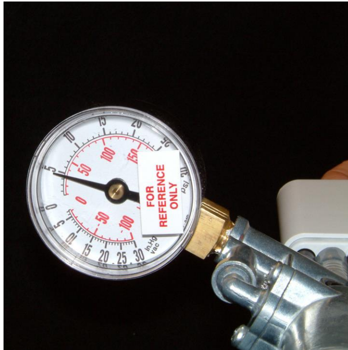
Figure 16 Pressure Pump at 4 psi
